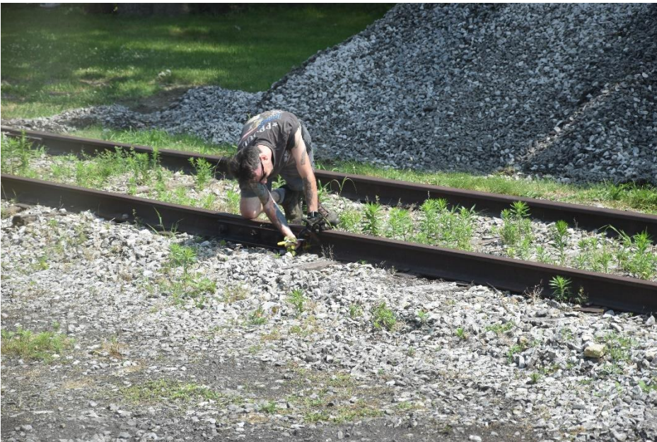
Bryce Dahl is marking rail as part of the siding reconstruction project. June 22, 2024.
